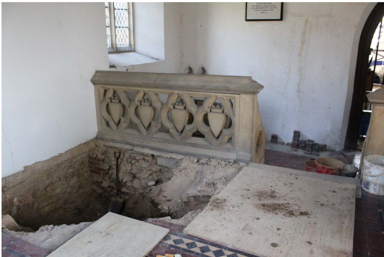
Subsidence in the raised floor of the Mausoleum 2010 due to inadequate structural compression
