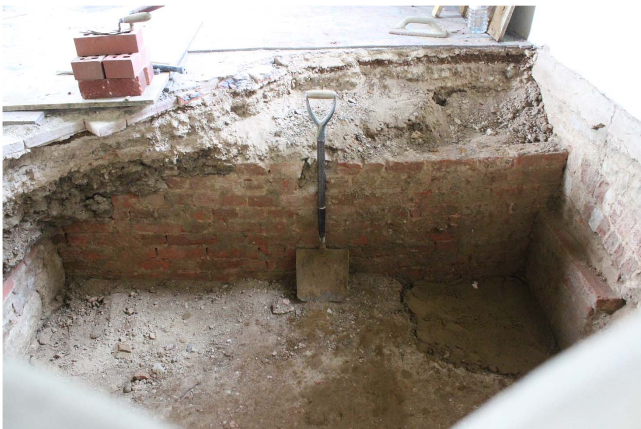
Blocking interior wall within Mausoleum revealed by sinkage of poorly compacted fill, 2010
